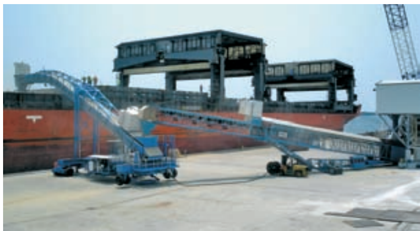
Shiploader with New Generation movement fed via Telescopic Link Conveyor
