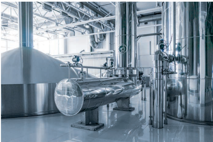
In the beverage industry, "Cleaning in Place" (CIP) is one of the standard cleaning methods for production plants. Pressure measurement plays a special role in this process
