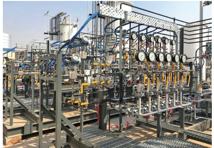
Chemical injection skid featuring six Proline Promass A 200.
