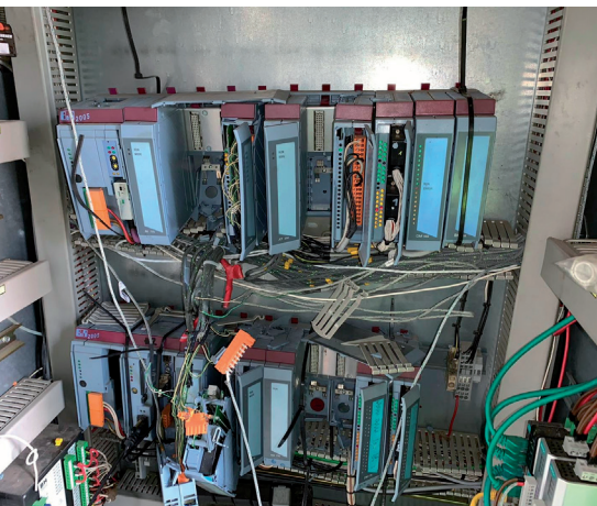
"Vandalised control panel and new Motortech panel after replacement."
