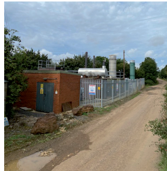
EDL's Wellingborough site
