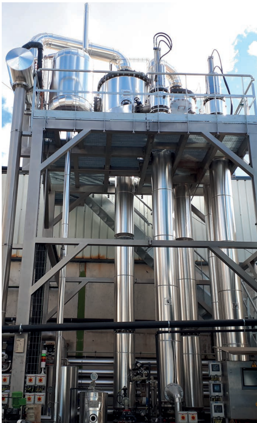
The ZLD system installed at Boxcapiel
