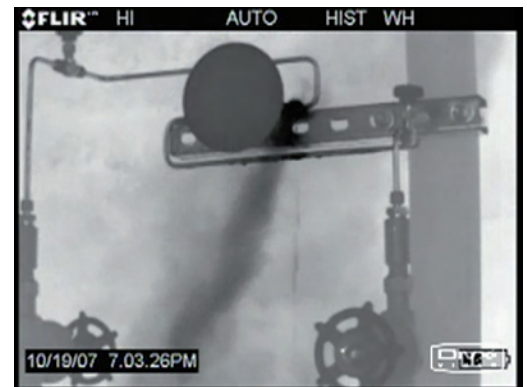
Recognizing leaks is the first step to reduce emissions to environment and save money
