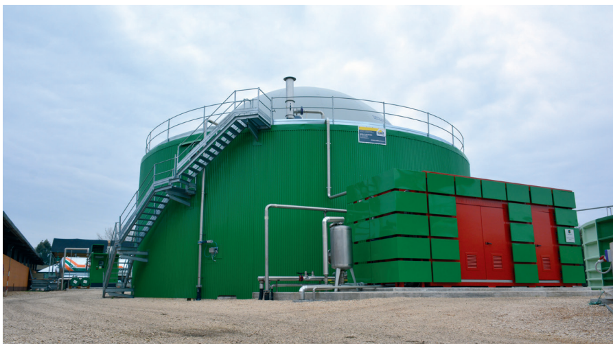
Roana has invested in a biomass plant that utilises livestock manure and other organic waste to generate energy. With it 2,400 kWh of electric energy can be produced every day.
