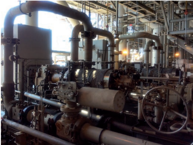
The tight confines around the injection pumps added to the challenges of the repair project.
