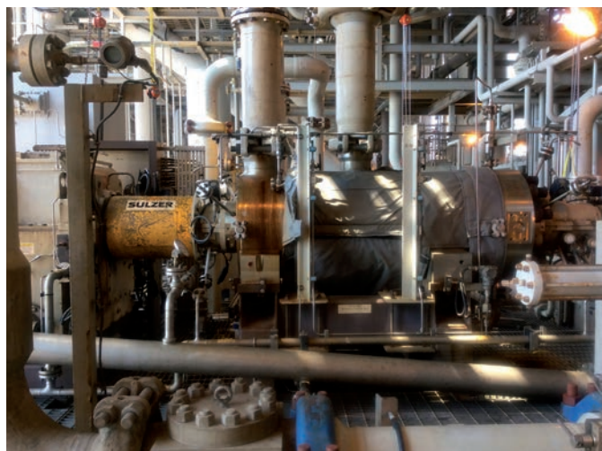
The water injection pump rejuvenated by experts from Sulzer.
