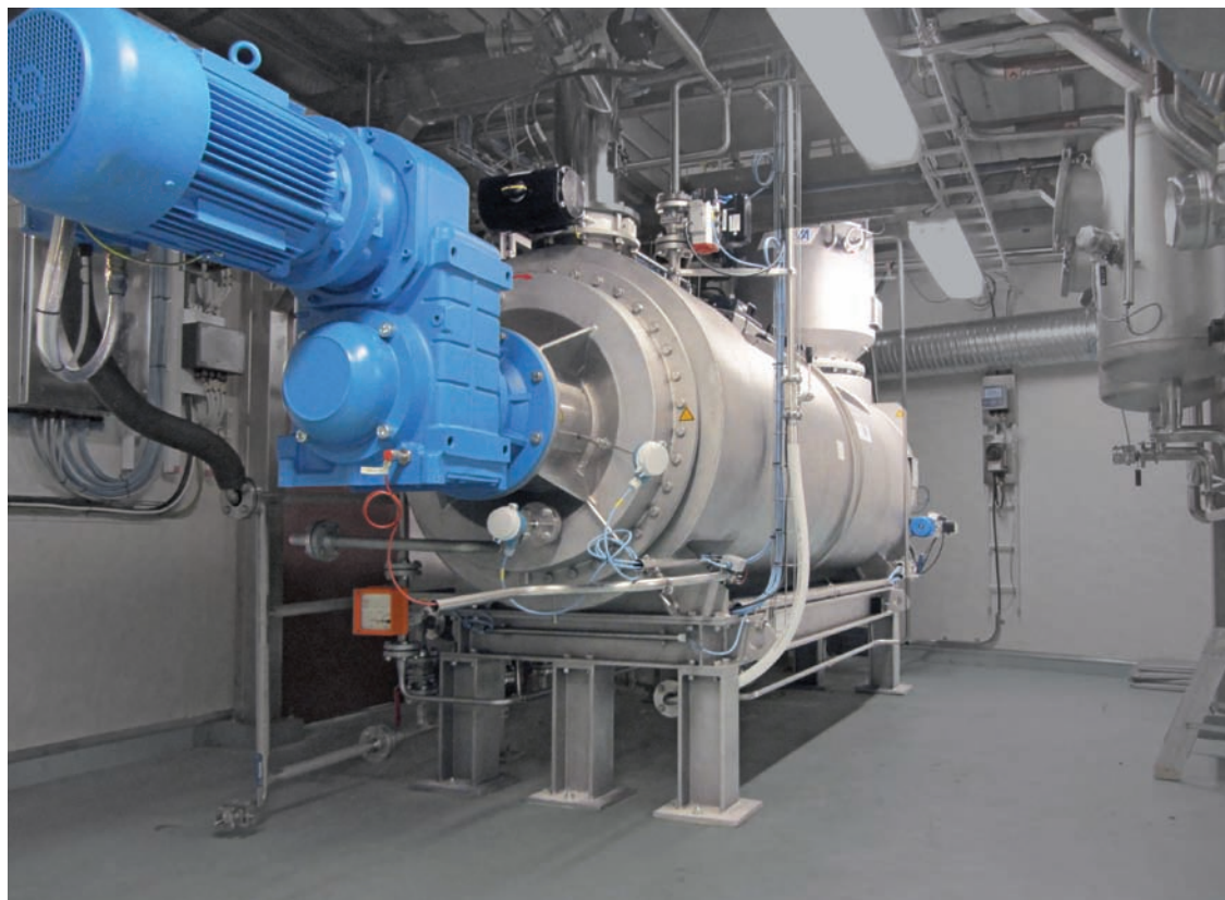
AVA installed an HTK-T continuous dryer for drying egg yolk powder
